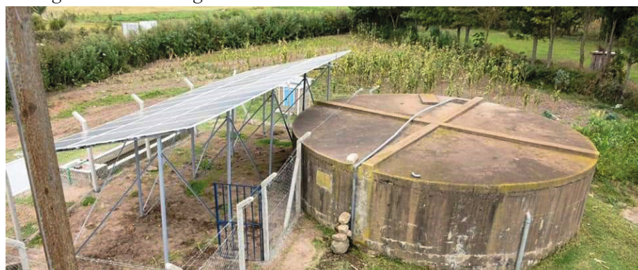
Solar Powered Borehole
