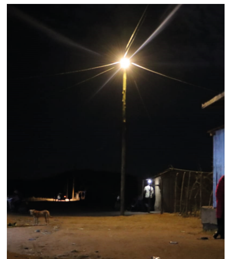
Street lights at Olderkesi trading center
